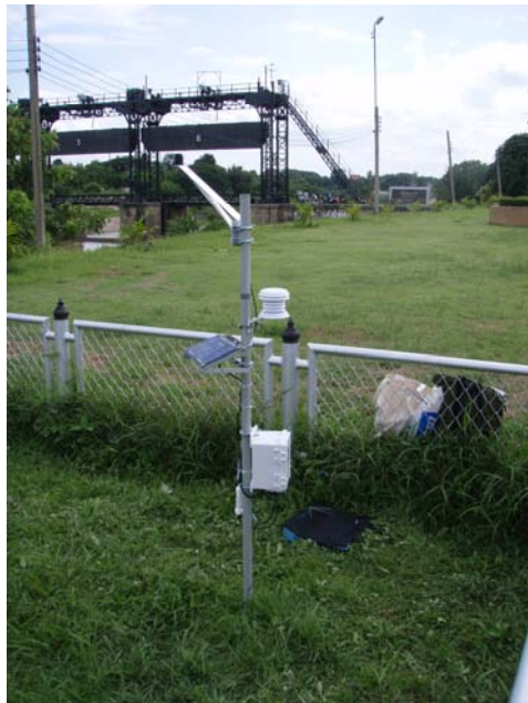
Fig. 16 A hydro-meteorological observation instrument installed at the Rama VI office, RID.
